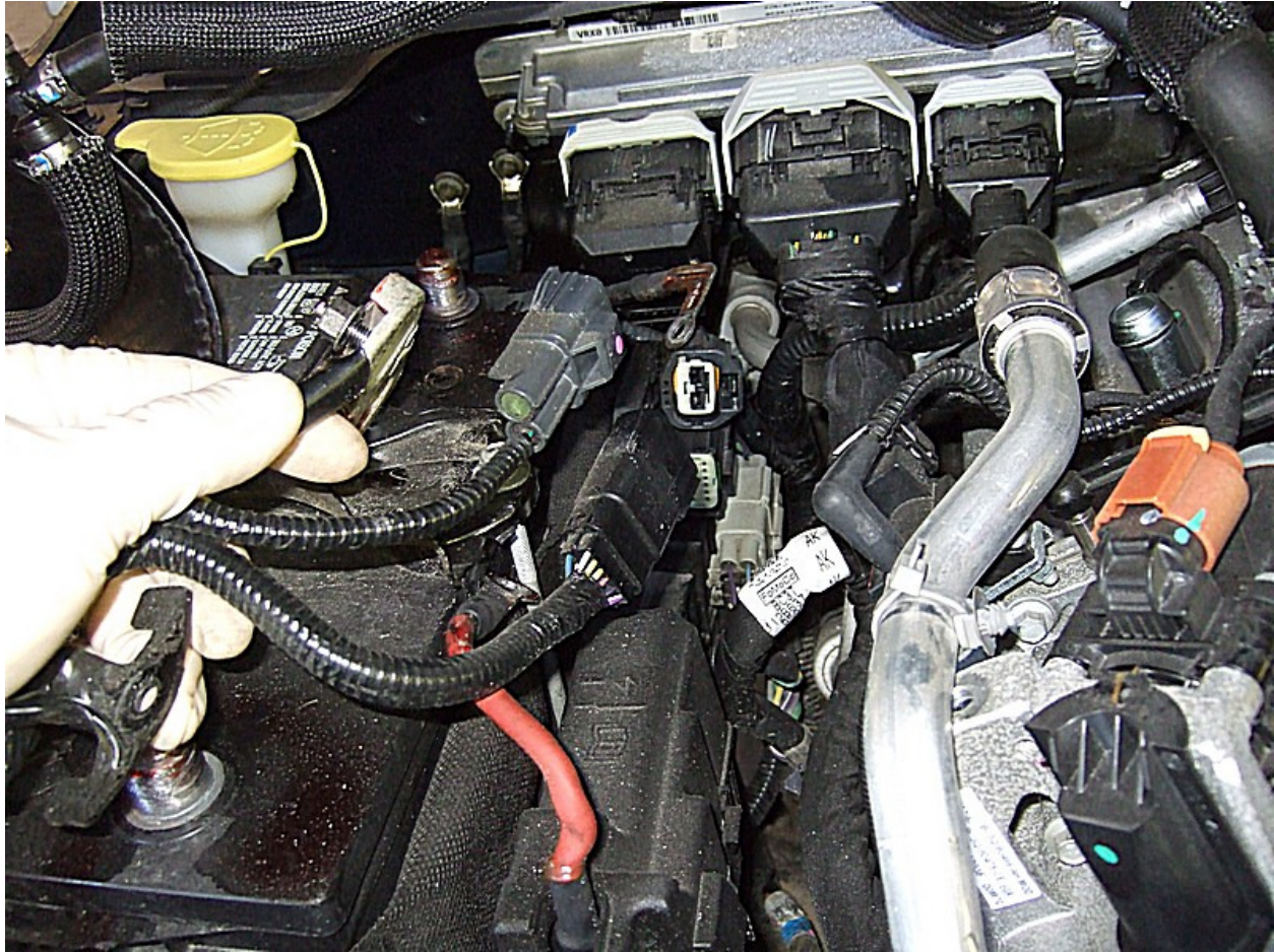
These two connectors are part of the battery cables, disconnect them. The cables are now free from the body and can be laid on the engine.
